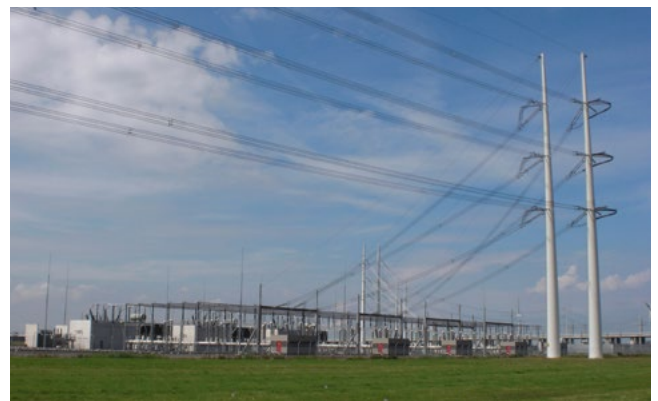
Netherlands: The TenneT Wintrack system reduces exposure to electromagnetic radiation by 60 %.
