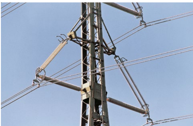
Worldwide First Braced Line Post for 420 kV in 1998
